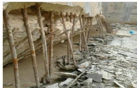
Gambar 1. Dinding WWTP rusak
