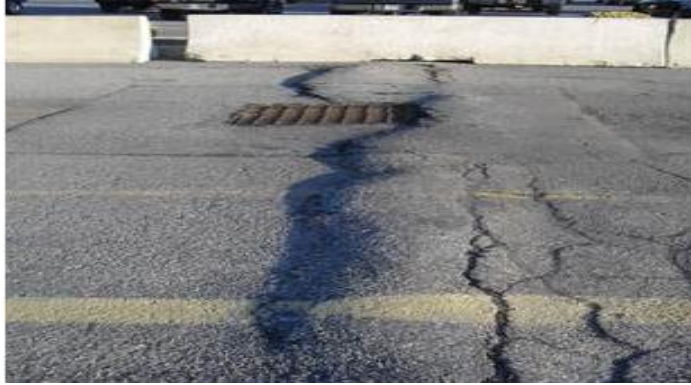
Gambar 2.18 Tonjolan dan Lengkungan ( Bumps and Sags ) Sumber: https://keselamatanjalan.wordpress.com/2017/12/26/jenis-kerusakan-jalan-lentur/
