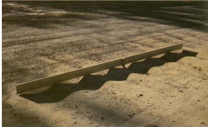
Gambar 2.11 Kerusakan Keriting ( Corrugation )
