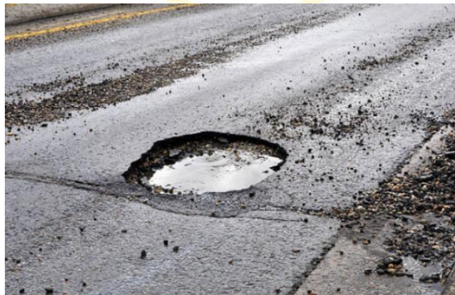
Gambar 2.15 Kerusakan Lubang ( Patholes ) Sumber: https://meonuk.com/blogs/news/how-do-potholes-form
