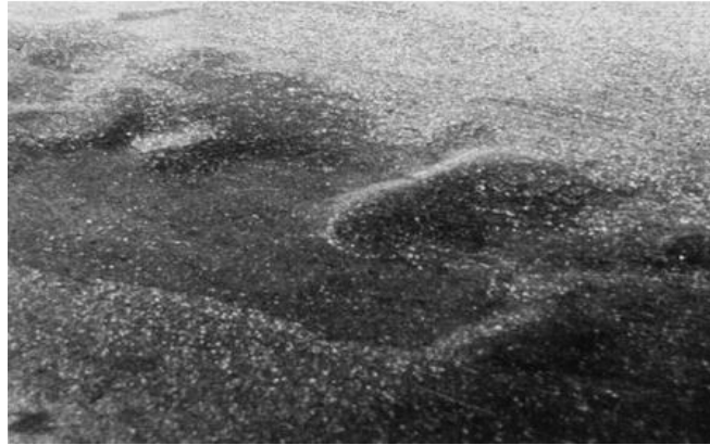
Gambar 2.12 Kerusakan Sungkur ( Shoving )
